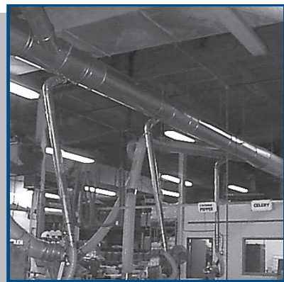
Straight duct from 3 to 24-inches diameter.
